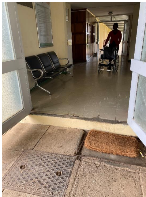
Proper ramp needs to be installed at the entrance
