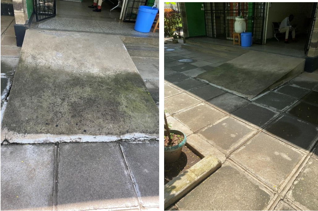
Accessible ramp however, it has no handrails.
